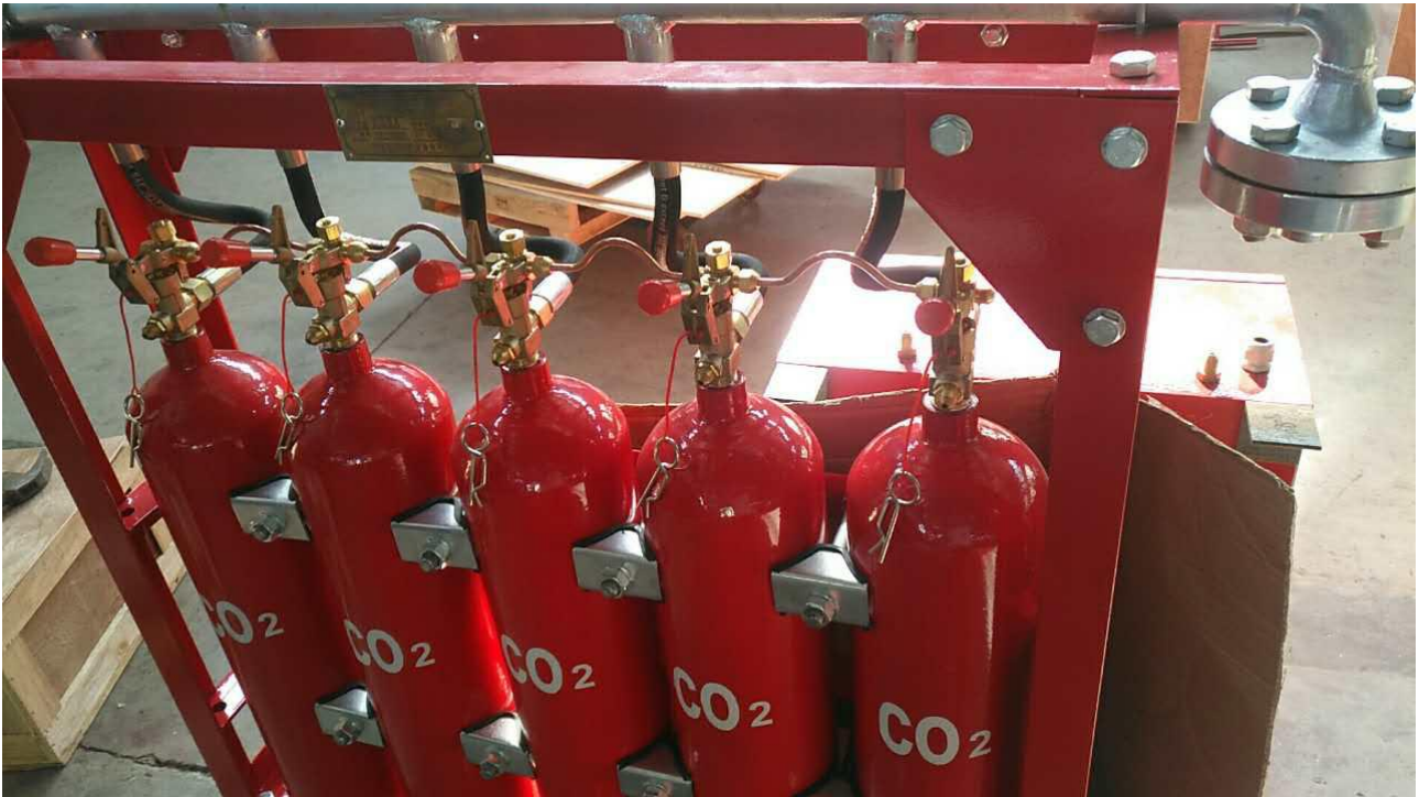
CO 2 Fire-fighting System
